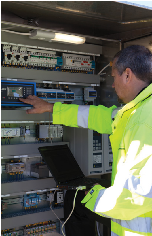
Smart pumping controllers can deliver significant improvements in performance
