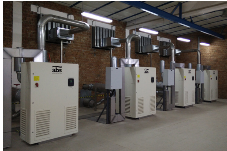
The new turbocompressors improve the efficiency of the Ostrowiec plant
